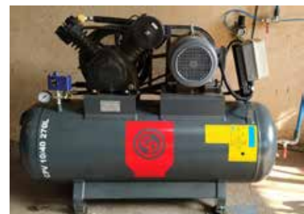
Compressor for Paint Shop
